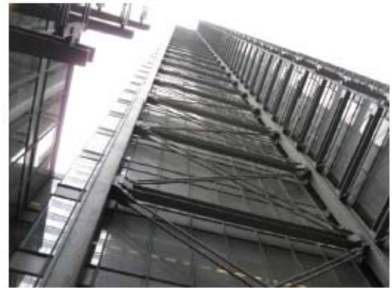
Figure 8: Image of Rod X-Braces at Notches
